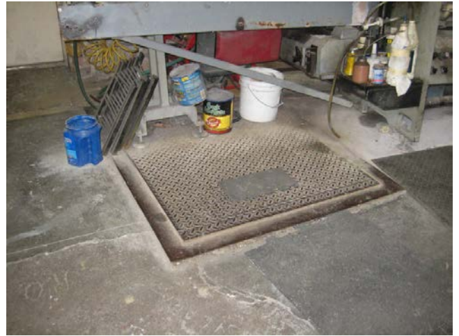
6. View of the oil/water separator.
