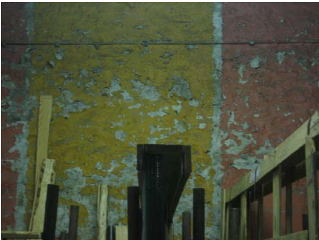
15. View of peeling wall paint inside the subject property.
