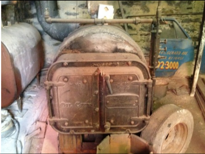
PHOTO 9: Looking at the dilapidated boiler within the building.
