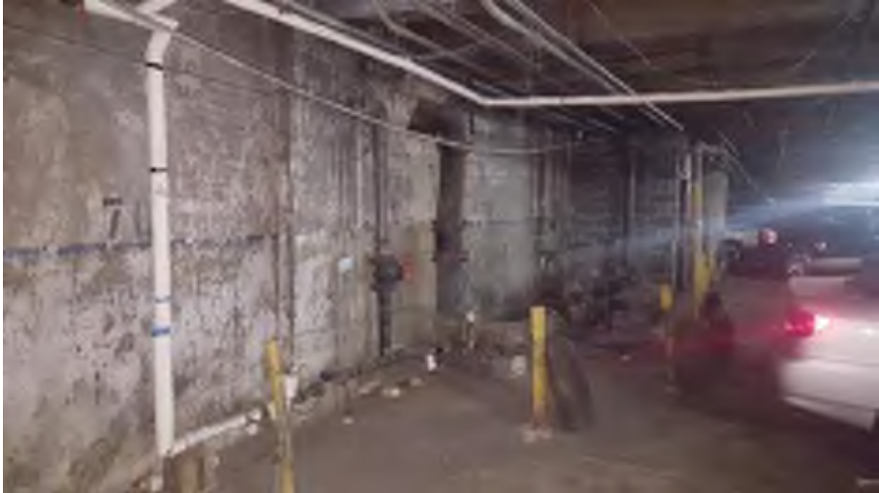
Photograph 19: Building utilities entering basement of Subject Property along Broadway.
