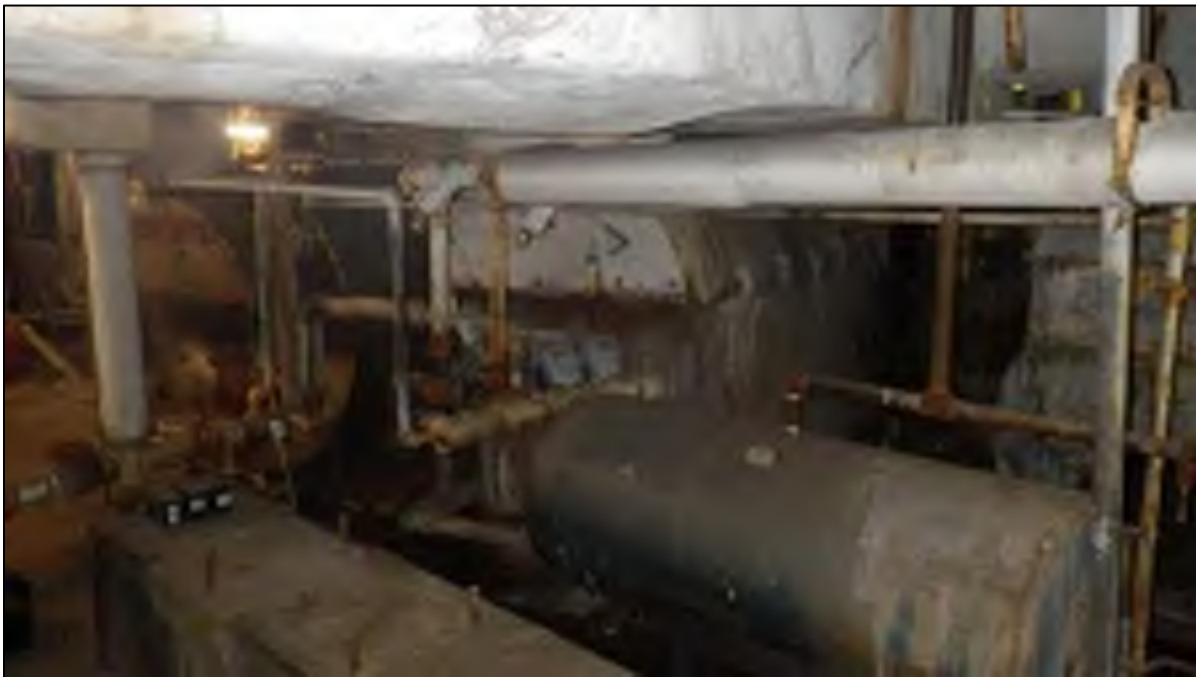
Photograph 4: View of boiler room within cellar.
