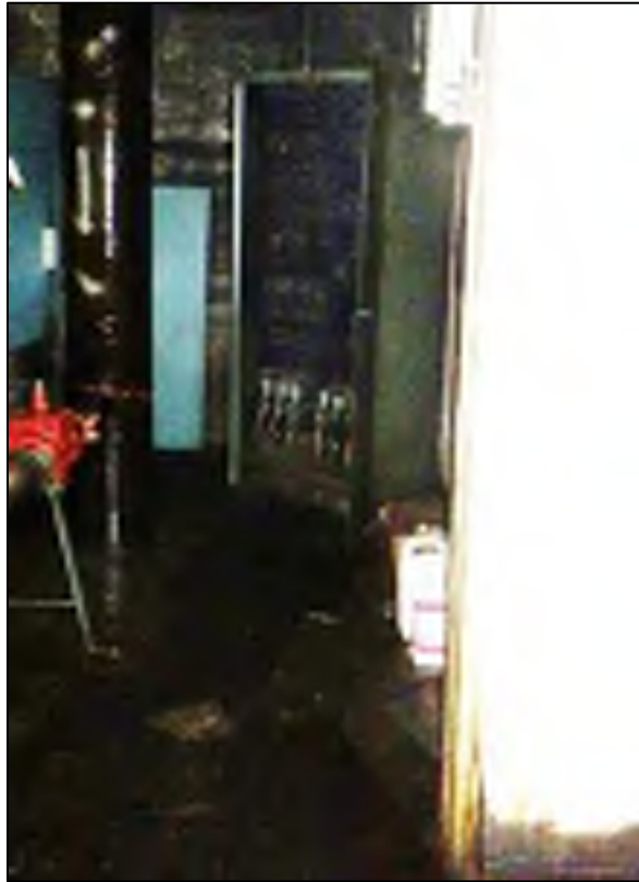
Photograph 5: View of hydraulic elevator room within the cellar.
