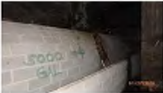
5,000-Gallon AST Encased in Concrete
