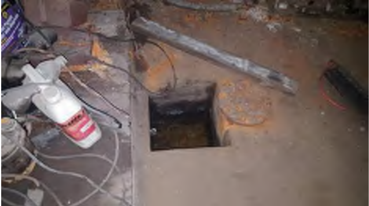
Photograph 23: Sump in sub-cellar boiler room.
