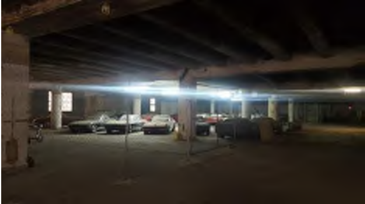
Photograph 7: Antique car storage on first floor of vacant northern portion of the Subject Property.
