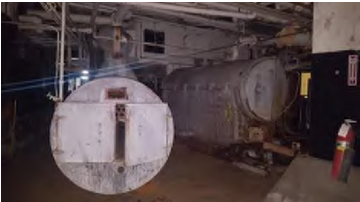
Photograph 20: Sub-cellar boiler room. Boilers are not functional.
