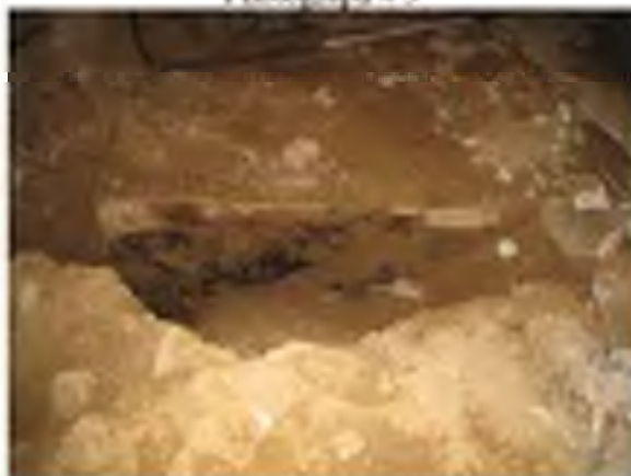
Steel USTs vaulted in concrete
