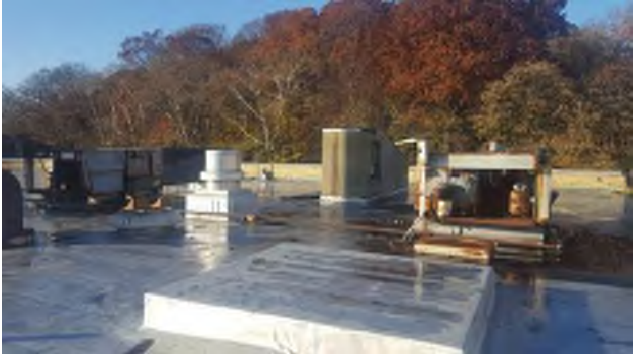
Photograph 3: Non-functioning heating, ventilation, and air conditioning (HVAC) equipment on rooftop.
