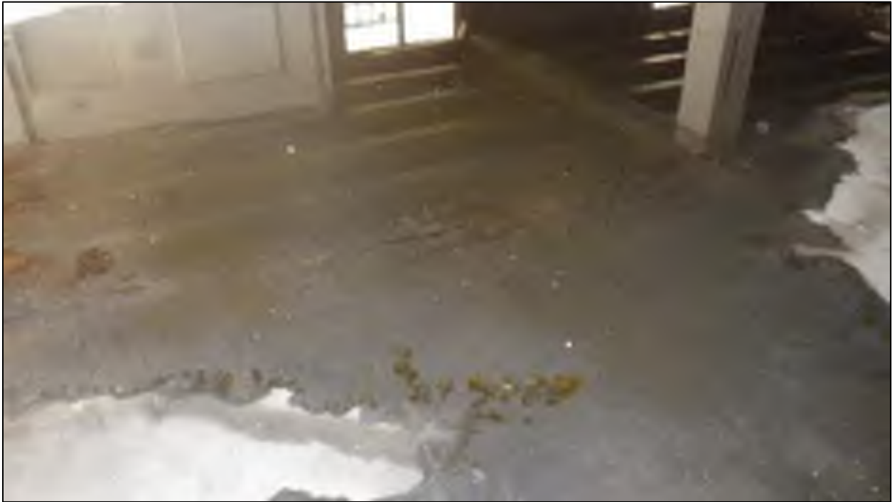
Photograph 11: View of standing water on floor of second floor.
