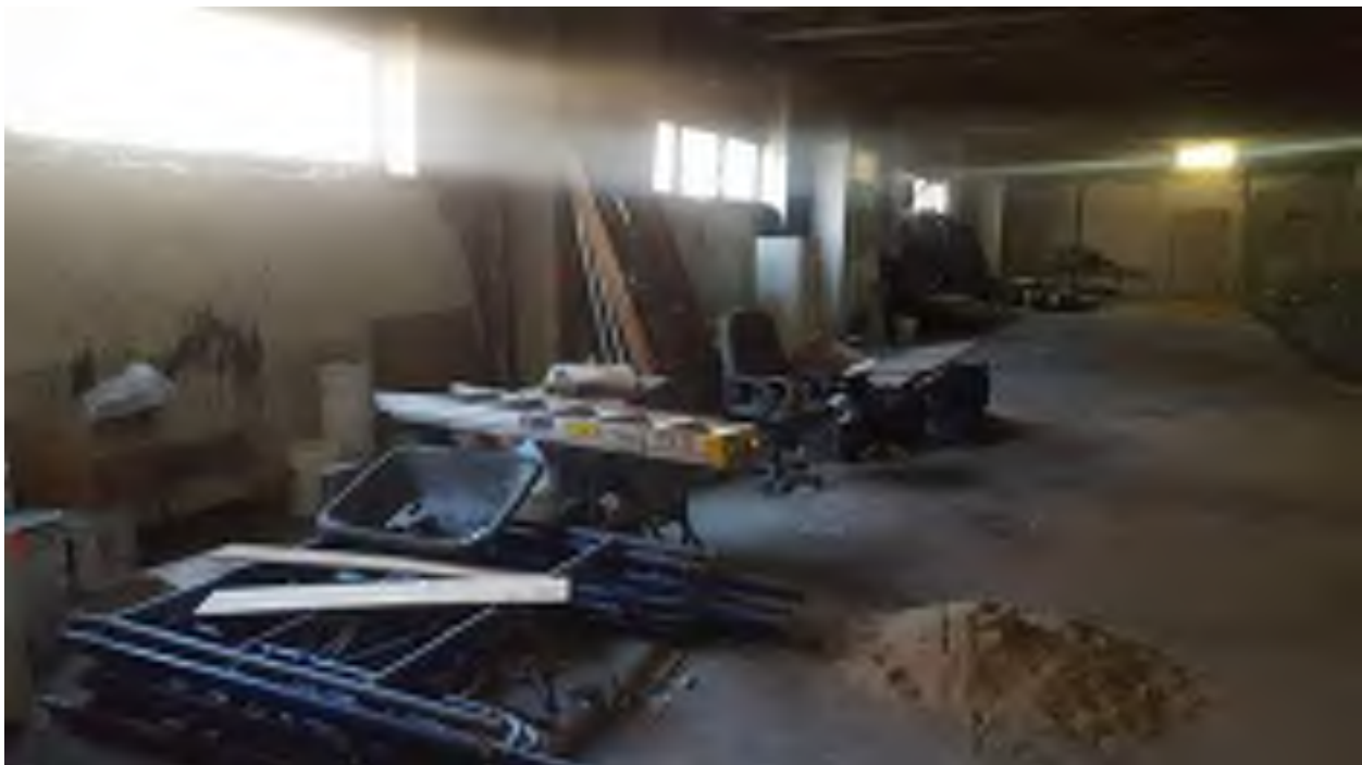
Photograph 8: Construction material storage on first floor of vacant northern portion of the Subject Property.
