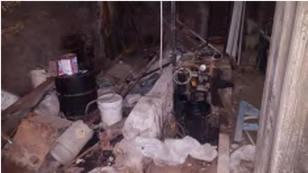
Photograph 22: Fuel pumps and staining in former tank room.
