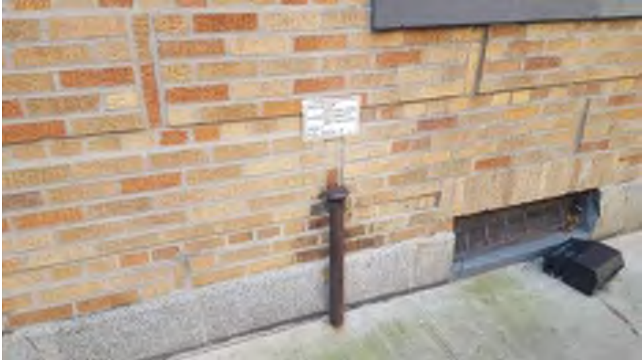
Photograph 33: Fuel oil fill port and vent pipe at northern adjoining property.
