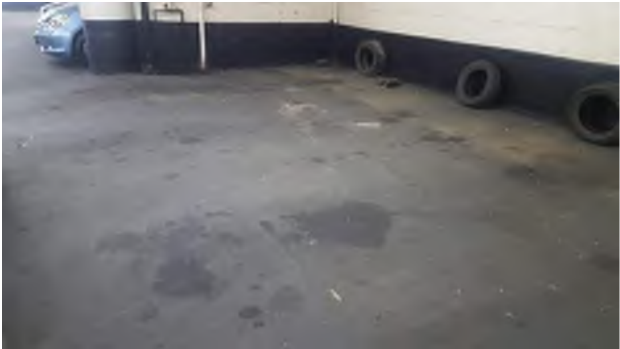
Photograph 24: De minimis localized staining across interior parking areas.
