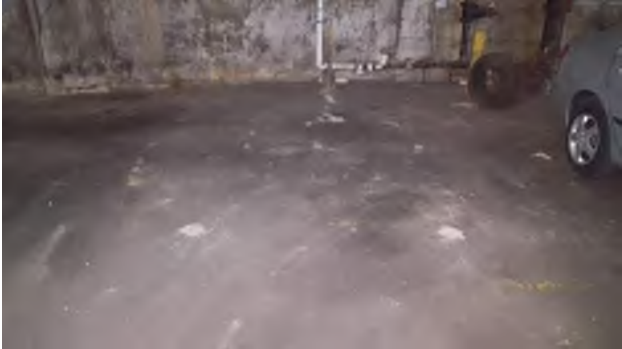
Photograph 17: Grouted borings shows evidence of subsurface investigation in southern area of basement.
