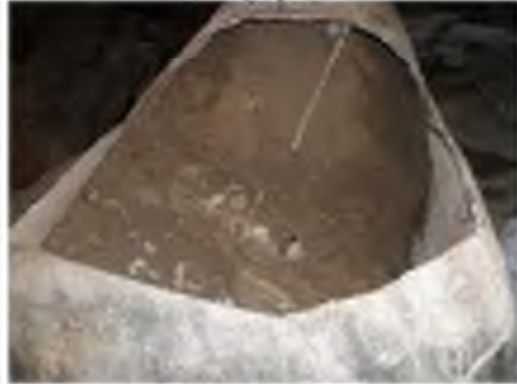
Sludge within UST
