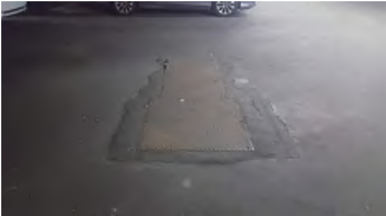
Photograph 18: Unidentified penetration in basement.
