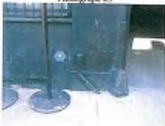
Vent Pipe for AST 4630 Broadway, New York, NY
