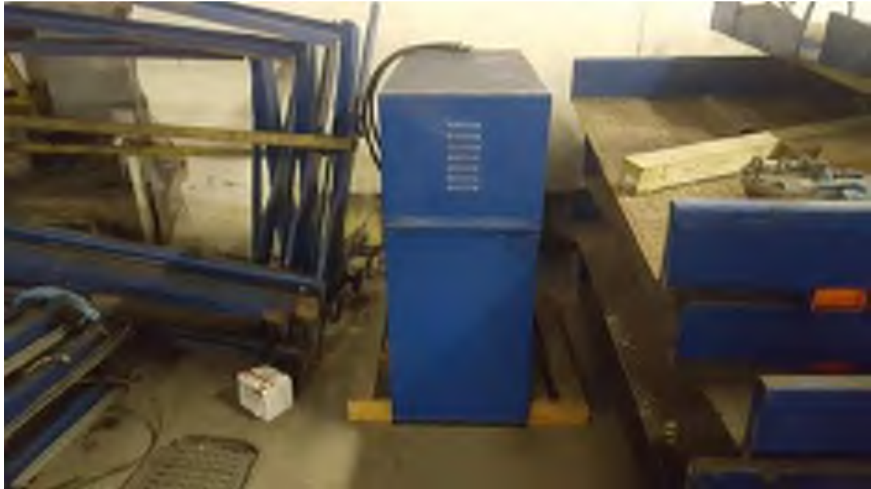
Photograph 11: Hydraulic tank and compressor for disassembled vehicle lifts.
