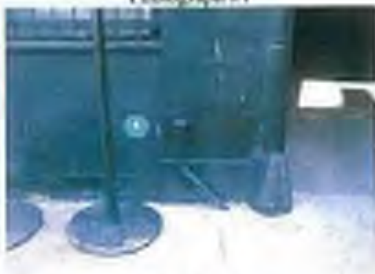
Vent Line Parking Garage 4650 Broadway, New York, NY
